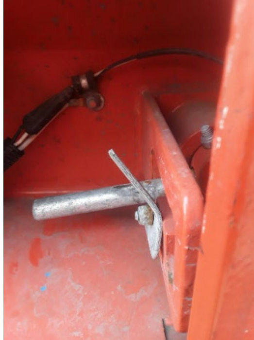
Bent or broken pin securement
